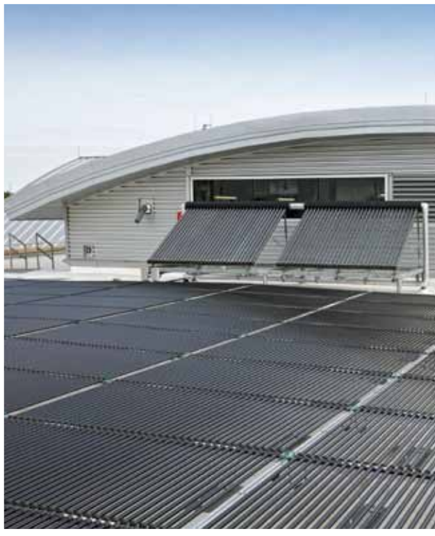
pictured above: Water Heating Tubes on the roof of Encore's newest building, The Research and Development Center, powered by our own photovoltaic wire
